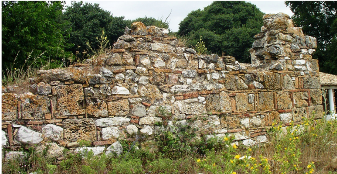
Fig. 107. Nea Sampsonda, Panagia sto Kozili, SW building. View of the E part of the S façade.
